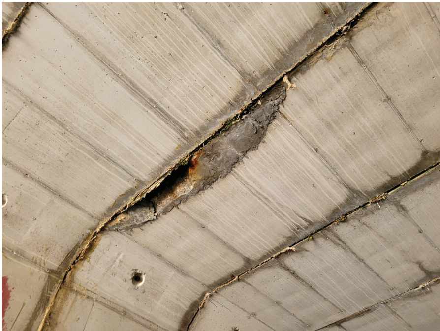
View of severe spall on central soffit.
