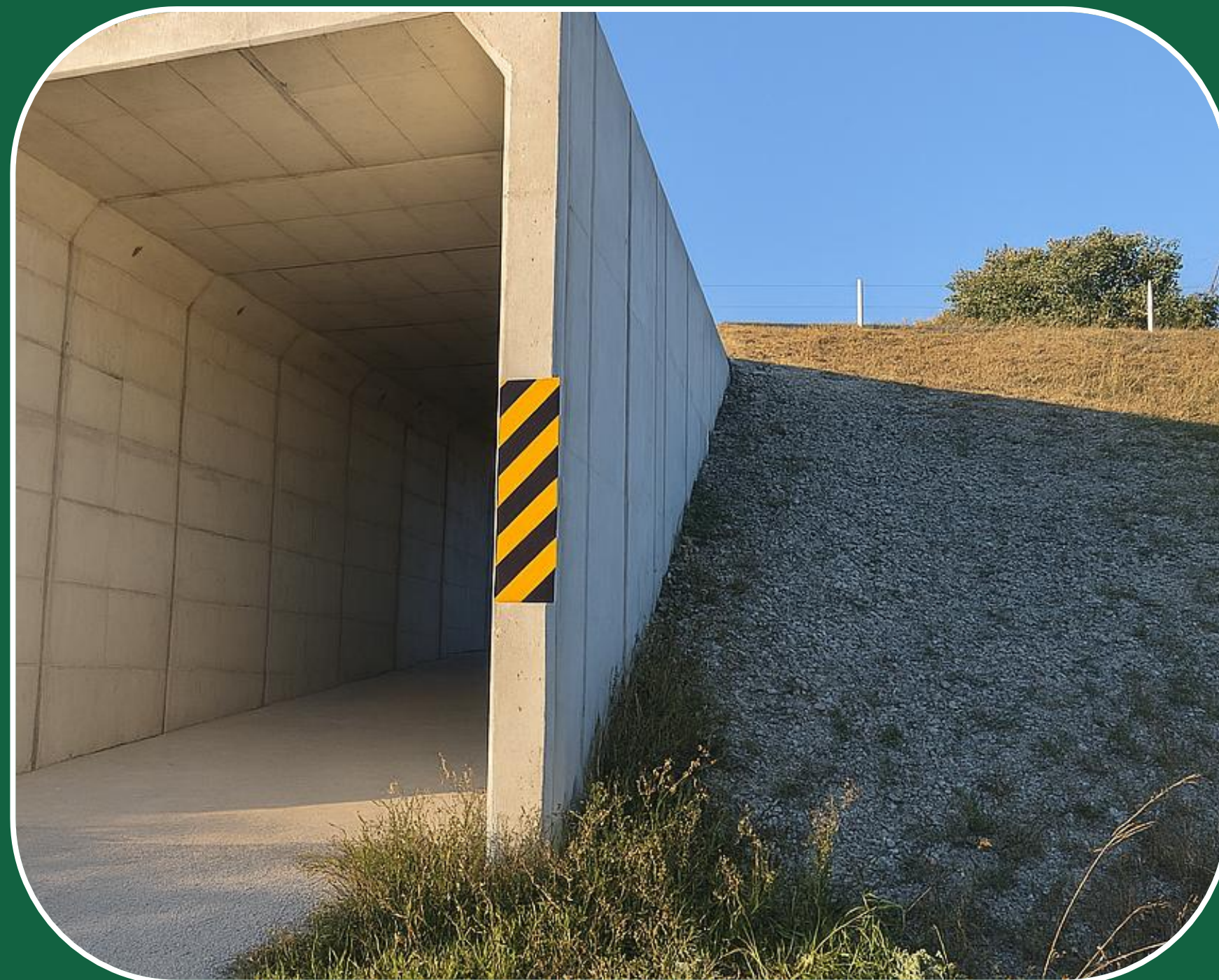
Replace Hazard Signs at Ends of Structure.
