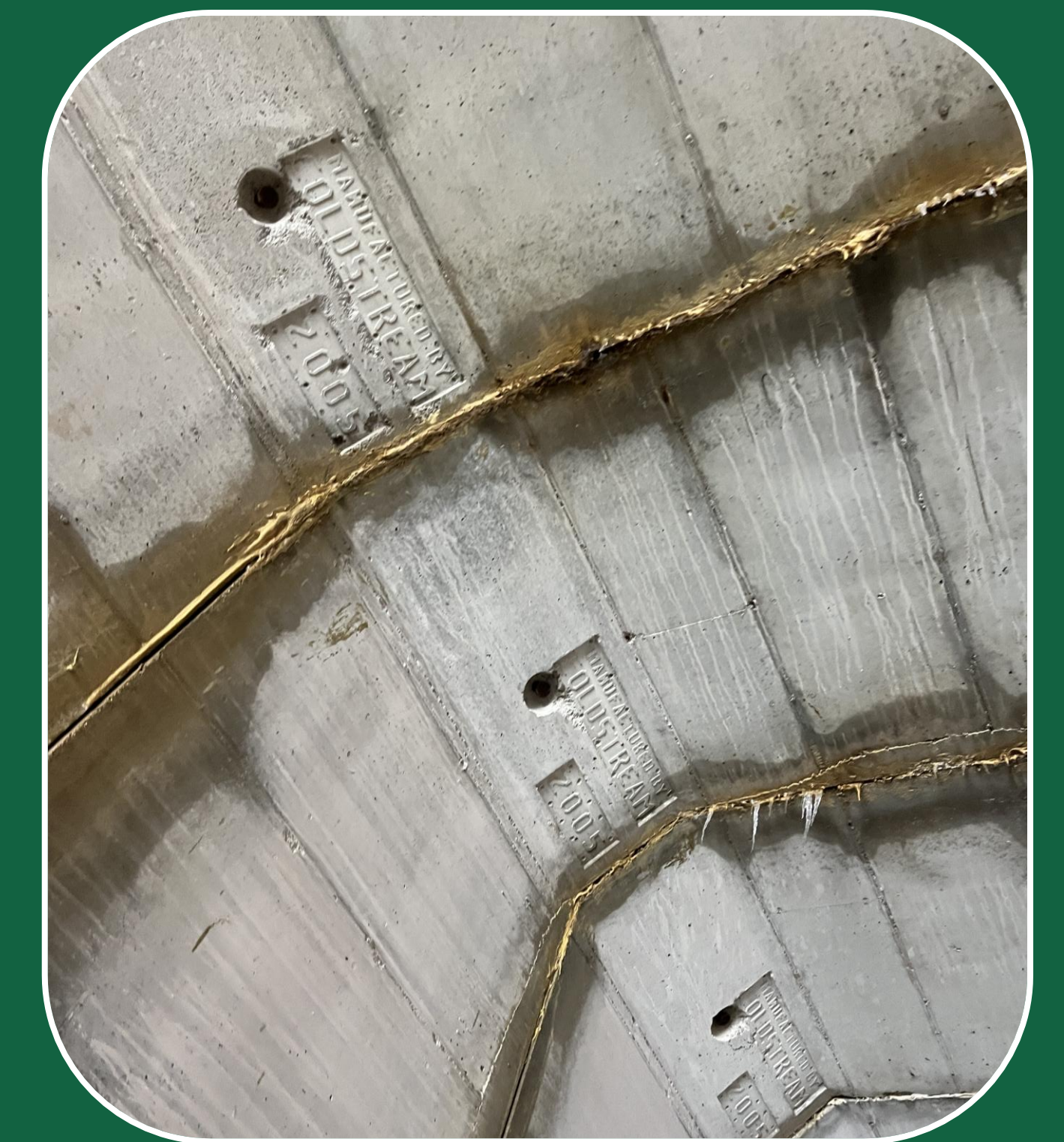
Water Infiltration at Interior Joints.
