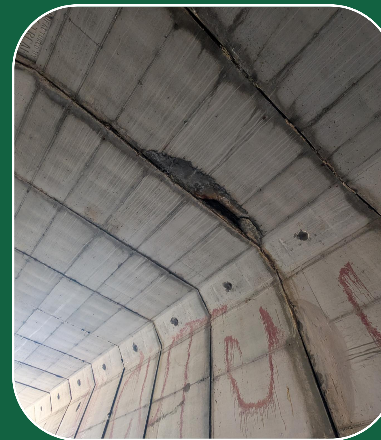
Spalling and Cracking at Interior Joints.
