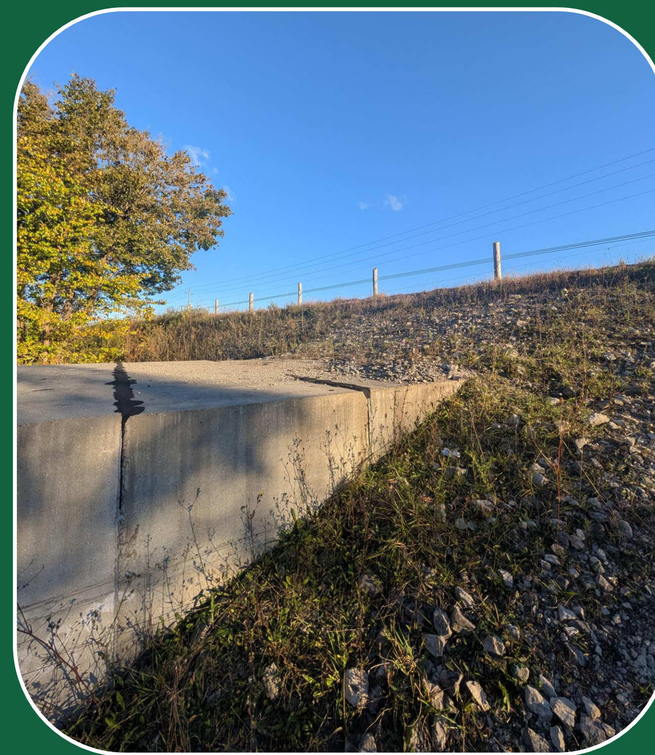
Exposed Deck Top and Loose Granular Embankments.
